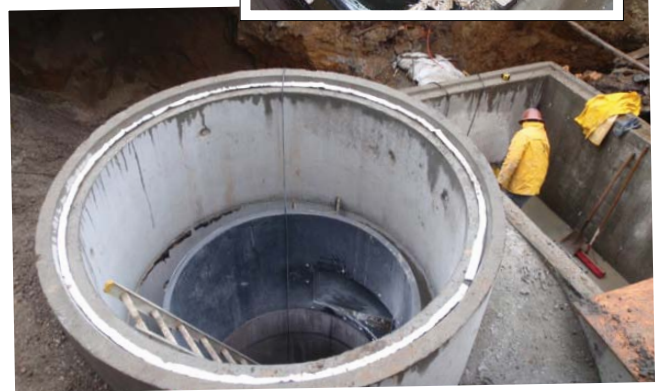
CDS unit installed to remove trash before entering Lake Meritt in Oakland, CA
